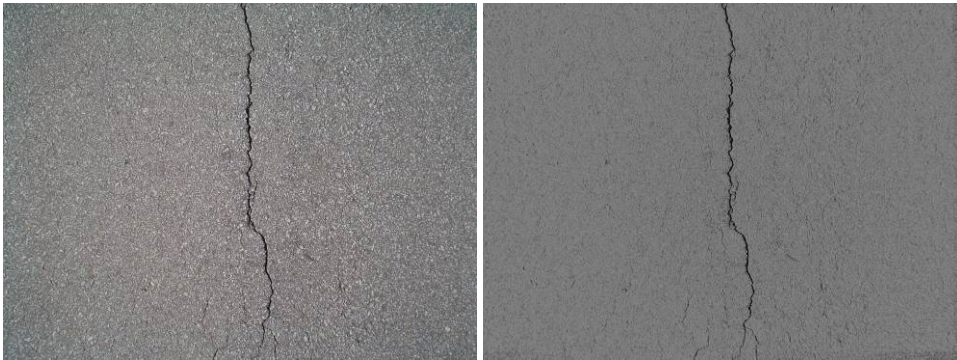
Fig. 7. Normalized image containing a longitudinal crack before (left) and after (right) applying the intensity saturation algorithm.
