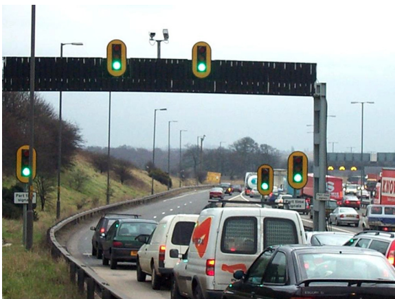
Figure 5.33 Ramp metering installation in the United Kingdom. Source: http://www.dft.gov.uk/itstoolkit/Tools/T33.php .
