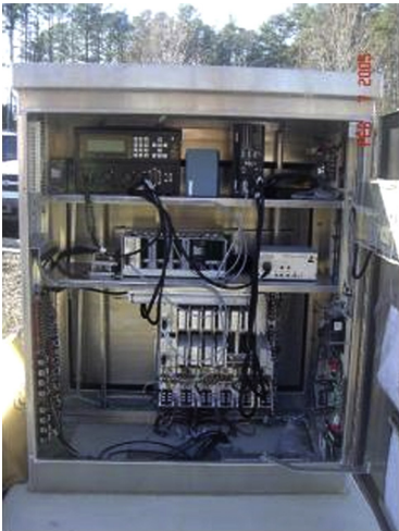
Figure 5.43 Signalized intersection controller. Photo by Chris Cunningham
