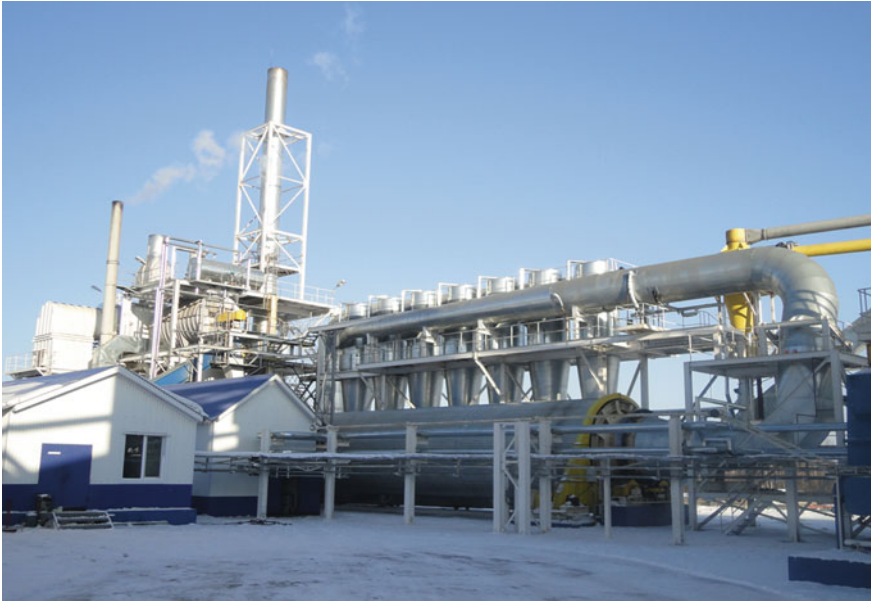
Fig. 6.32 Drum dryer for drying wood chips
