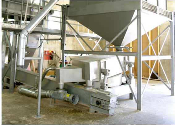
Fig. 6.61 Screen below the pellet cooler by Knoblinger [5]
