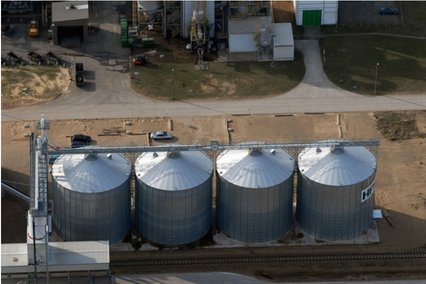
Fig. 6.62 Sheet-metal silos for pellet storage with feed and discharge conveyor and loading station
