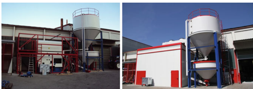
Fig. 7.28 Pellet boiler based on a 1,000 kW feed grate firing system with adjoining pellet silo by Kohlbach, Austria [15]
