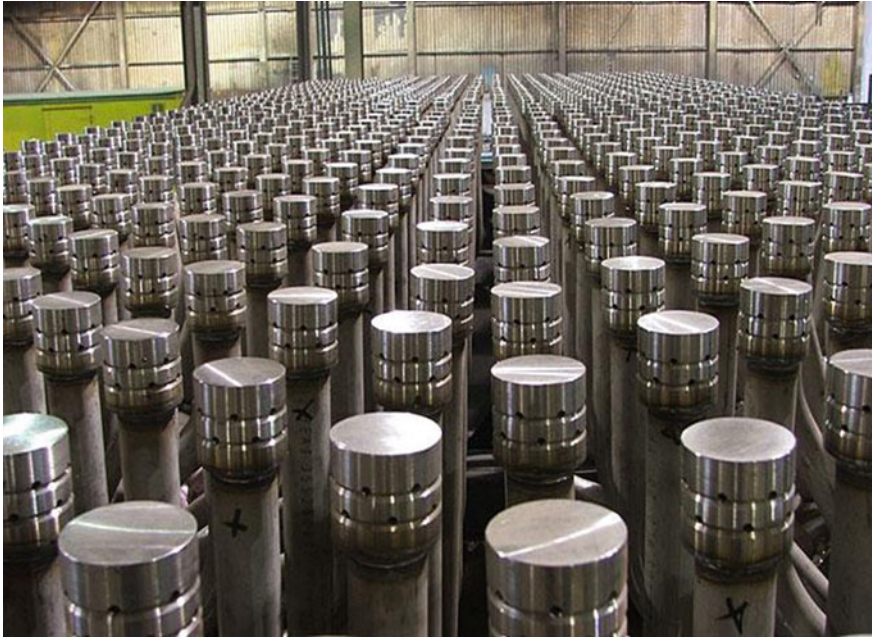
Fig. 7.33 Nozzle floor of a fluidized-bed firing system [16]
