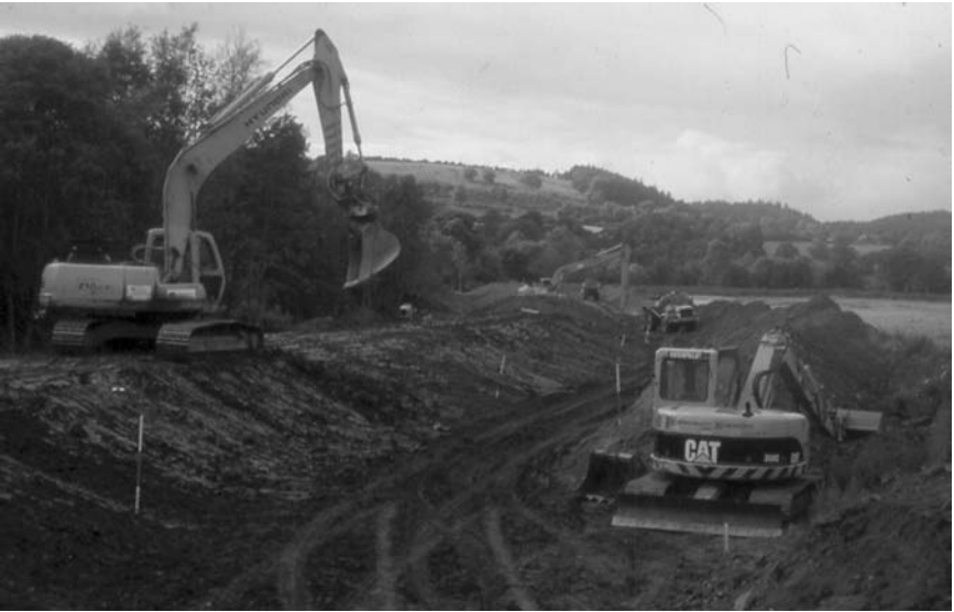
Plate 7.2(a) 'Making space for water': reinstatement of a flood bank to protect a recently damaged rural community – higher, stronger, but further from the river: removal of the old flood bank.
