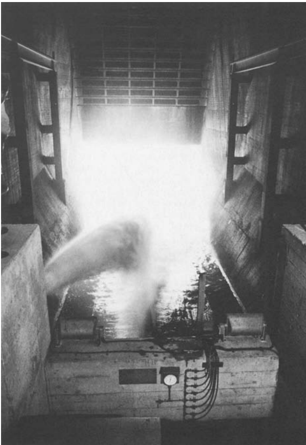
Plate 6.3 The control of river flows by valves: inside Clywedog dam, mid-Wales, regulating the flow of the River Severn (photo M. D. Newson).
