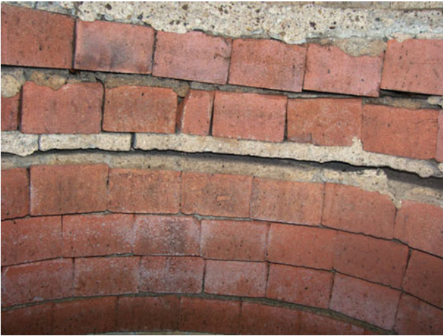
FIGURE B-2. Cracked Chimney.
