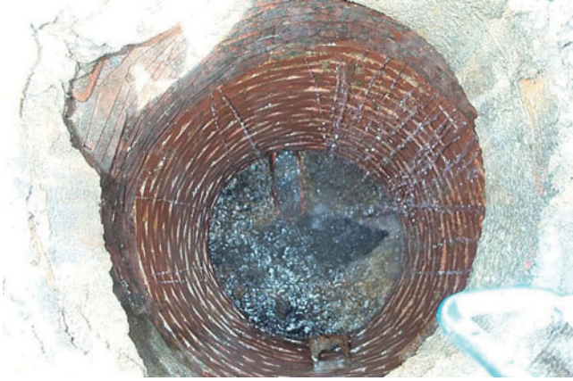
FIGURE B-5. Groundwater Infiltration through a Manhole Wall.
