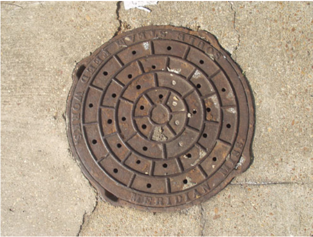
FIGURE B-4. Vented Manhole Subject to Ponding.
