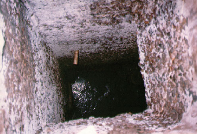
FIGURE B-3. Severe Hydrogen Sulfide Corrosion.
