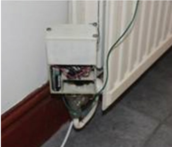
Fig. 13.6 Radiator valve in place
