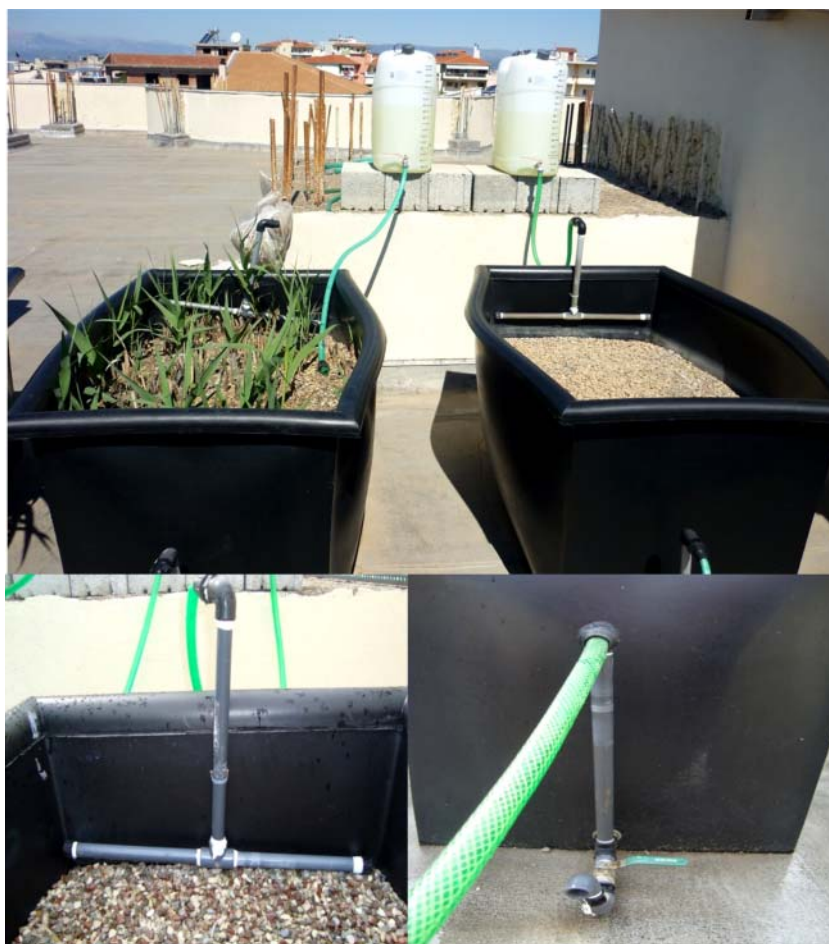
Figure 16.1 Pictures of the pilot-scale constructed wetland units.
