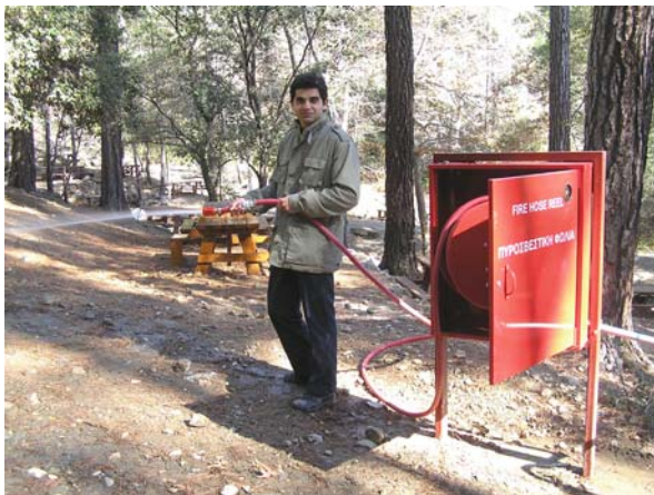
Plate 9 Risk index for fire management Fire reel hose system in picnic sites in Cyprus (Kazafaniotis), see box 19
