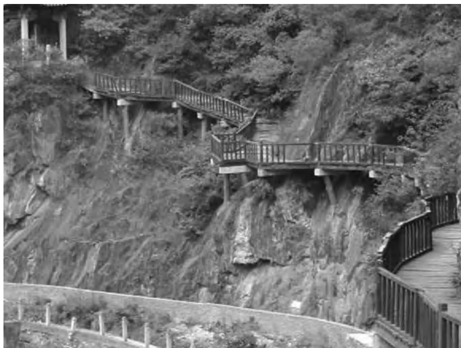
Figure 2.2 Stretch of trestle road ( zhan dao ) cut into the rock face, Sichuan.
