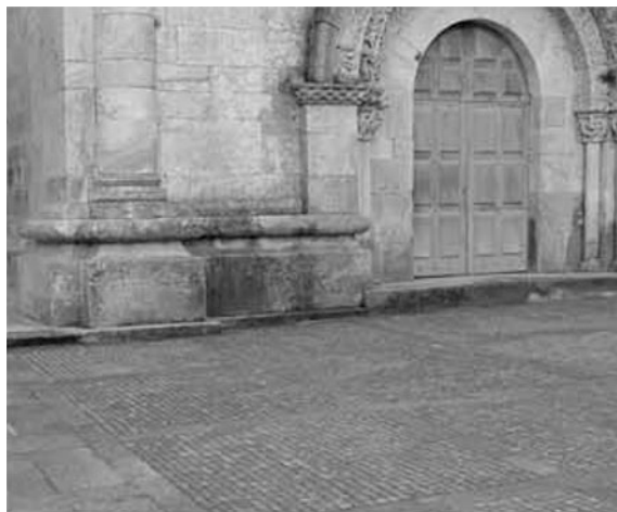
Fig. 2.2 Example of rising damp in a historical building
