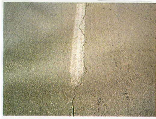
Figure B.2 Cracking – Severity Level 1
