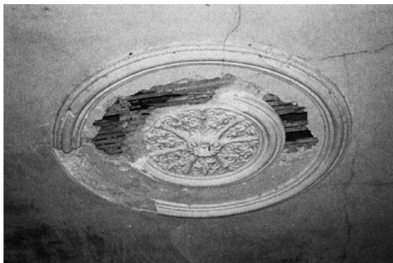
Fig. 9.10 Falling parts in decorative gypsum plaster piece (Pacheco-Torgal and Jalali 2009b)
