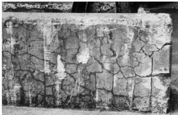
Fig. 9.3 Concrete cracking due to ASR
