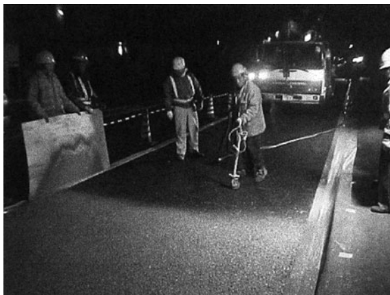
Fig. 10.8 Using \text{TiO}_2 photocatalytic material on roadway for pollution reduction (Fujishima et al. 2008)
