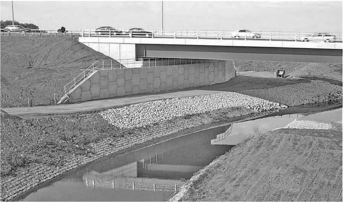
Figure 3.4 The River Blythe Bridge: view of semi-integral abutment and weathering steel girder
