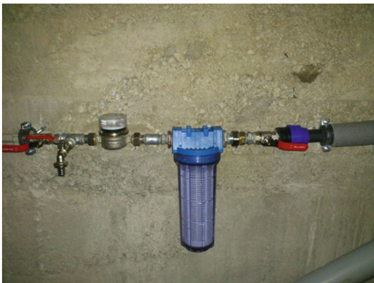
Fig. 4 Connecting pipes, filter, and water meter
