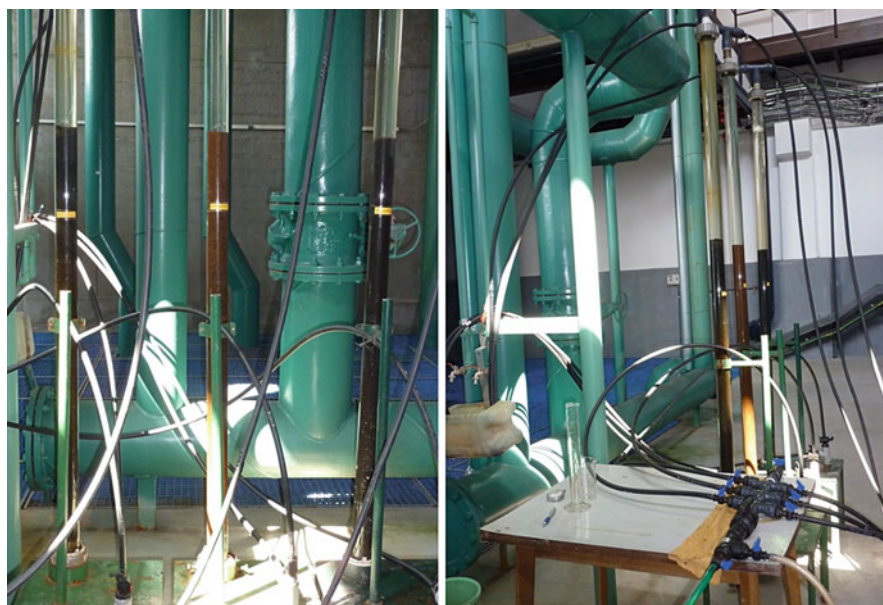
Fig. 15 Filtration equipment – filtration columns
