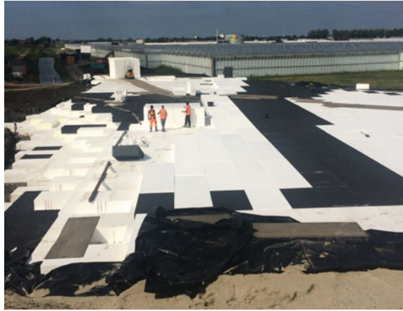
Fig. 4 Lightweight EPS-geofoam embankment (in the north) of the access road and the roundabout of the N222
