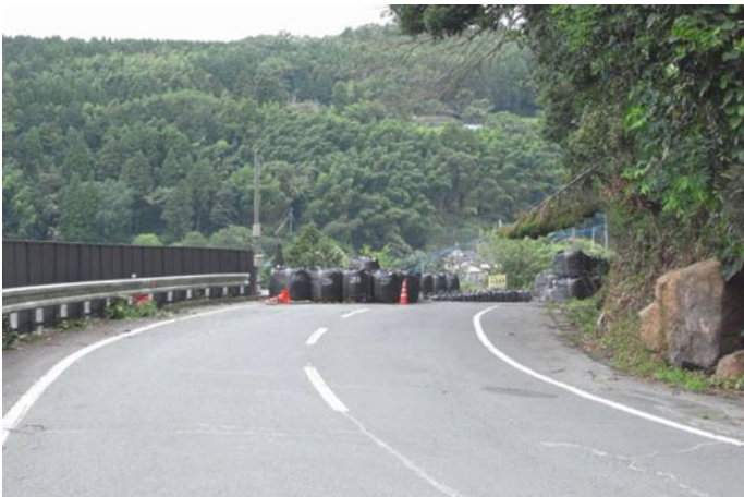
Fig. 10 Remediated surface of collapsed EPS embankment with restricted road width
