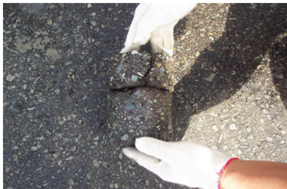
Fig. 2 Drilled cores on the cracked pavement above EPS
