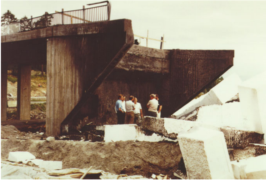
Fig. 34 Bridge abutment damaged by EPS blocks put on fire (NPRA)
