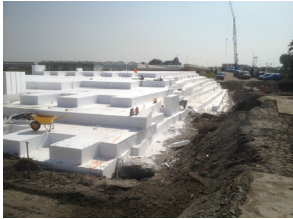
Fig. 5 Visible EPS fill belonging to the lightweight N201 road embankment nearby the aqueduct
