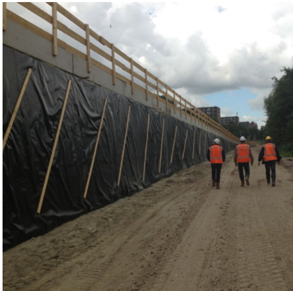
Fig. 6 The EPS fill (covered temporarily only with a membrane) with virtually vertical sides
