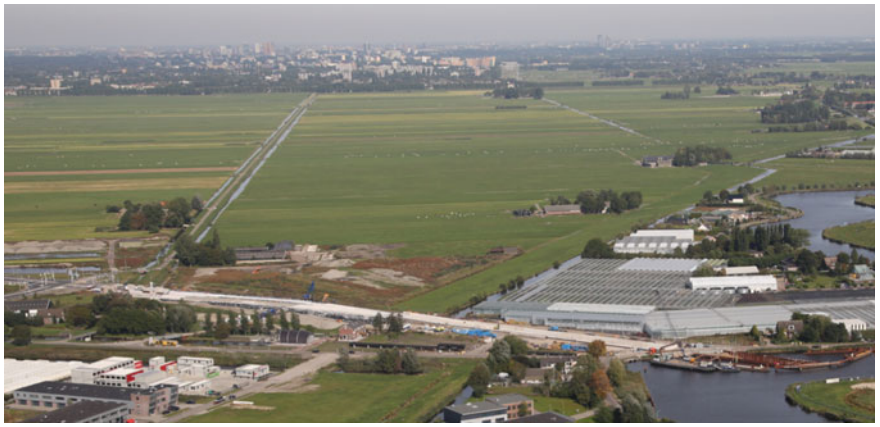
Fig. 2 Lightweight embankment of the provincial road N201 nearby Uithoorn and the aqueduct under the Amstel River under construction
