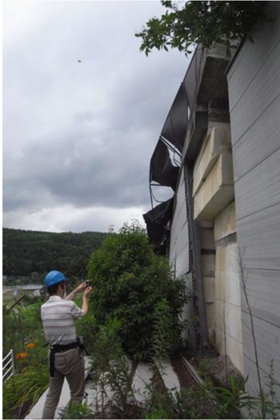
Fig. 4 Collapse of outer protective wall
