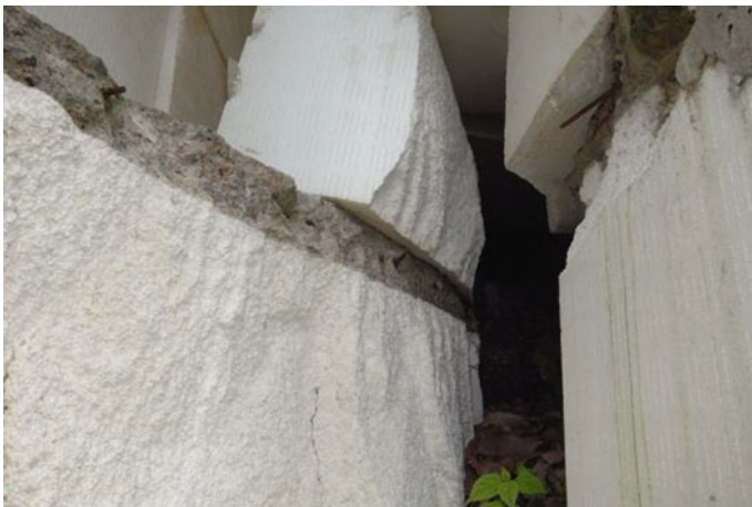
Fig. 7 Crack in intermediate concrete slab
