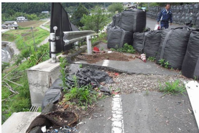
Fig. 2 A 1-m-wide crack in the road surface after refilling
