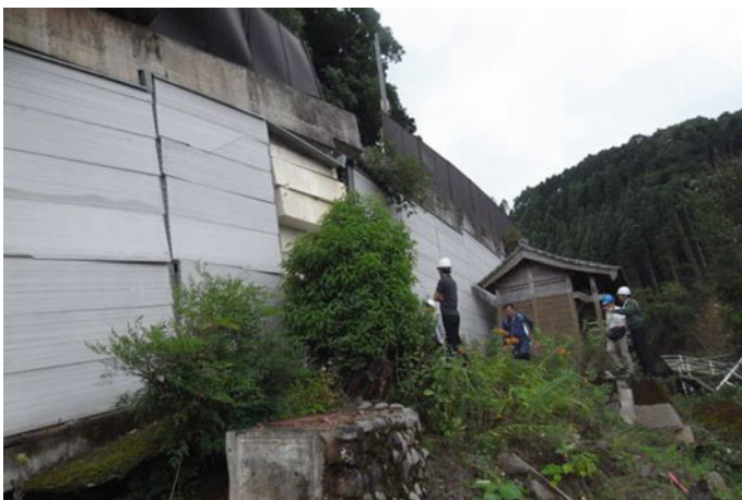
Fig. 1 Deformation of EPS embankment seen from the temple side
