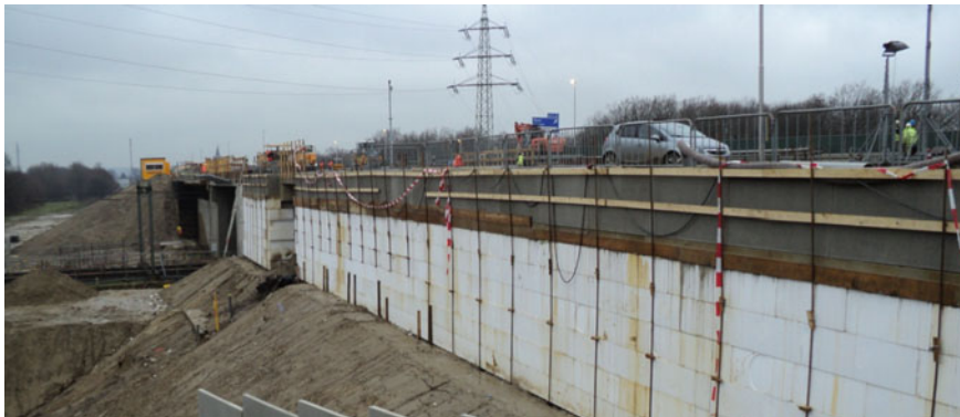
Fig. 5 The highway widening of the A76 with the not yet covered EPS side; The EPS bulk is piled up 4 m above the slope line; the truncated slope is supported by an existing retaining wall. The new concrete wall in the foreground has only a shielding function for the EPS construction in case of calamities from the Chemelot terrain
