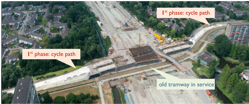
Fig. 4 The first autonomously completed embankments cross section part for the bicycle cycle path/road construction over the future motorway A4
