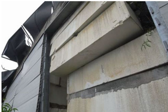
Fig. 5 Displaced EPS blocks
