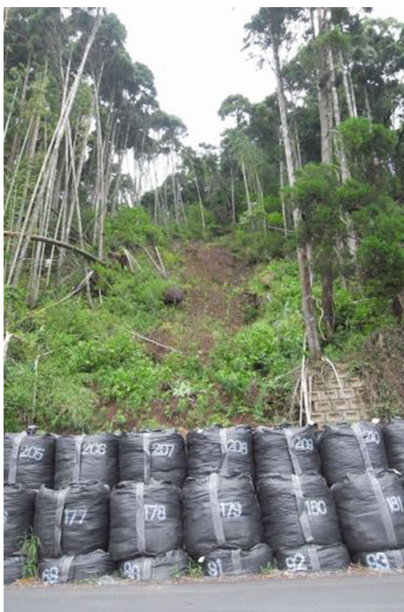
Fig. 3 Collapse of rear slope and temporary remediation
