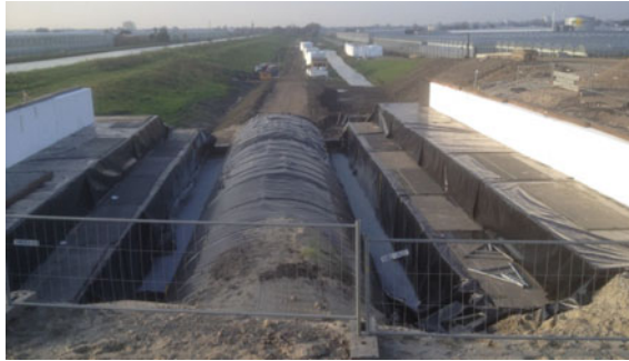
Fig. 8 The corrugated steel sheets covered by the membrane before pouring the foamed concrete enclosure of the cycling tunnel
