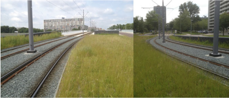
Fig. 7 Evaluation photos prove that no settlement differences have occurred after four year in service of the lightweight embankments with the tramway tracks and the cycle path/calamity road construction
