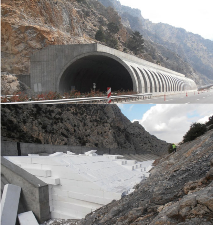
Fig. 23 Geofoam blocks applied for energy absorption on rock fall protection tunnel in Turkey (Courtesy of EPSDER, Turkey)
