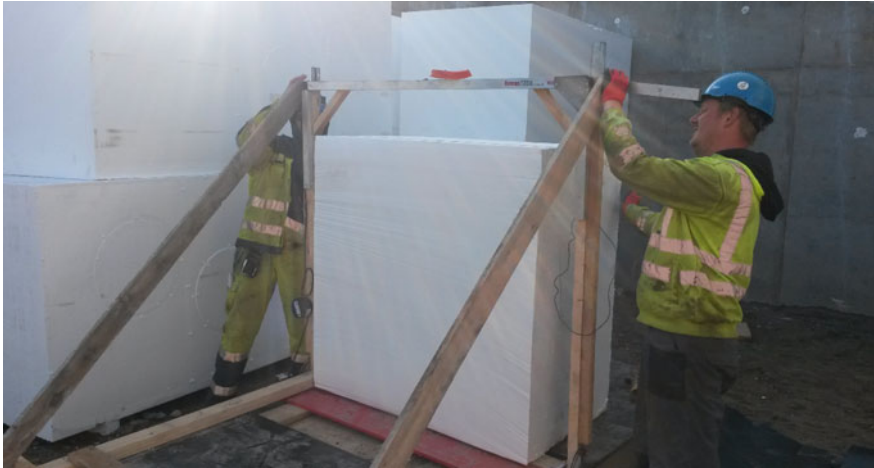
Fig. 5 Cutting the EPS geofoam blocks with hot wire apparatus at the construction site
