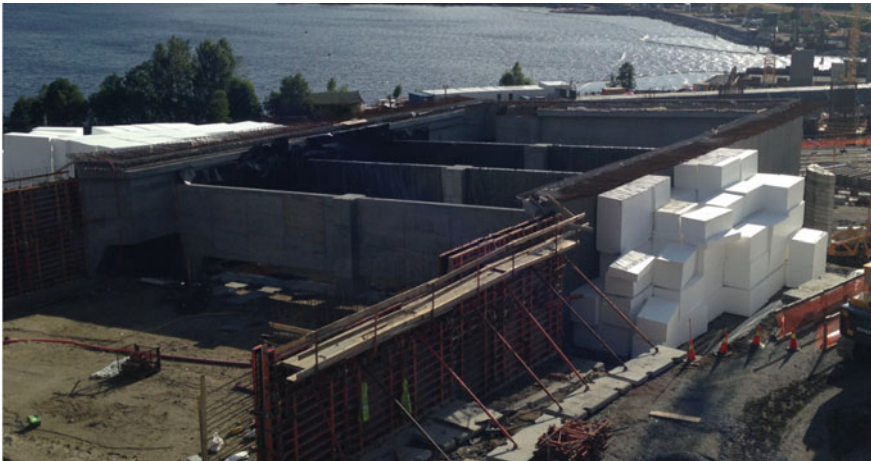
Fig. 4 Crossfall of 7.5% for the roadbed and storage of geofoam blocks at the construction site
