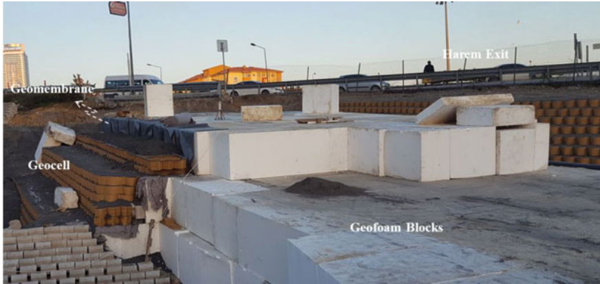
Fig. 4 Geomembrane protection and geocell application at the sloped section of the geofoam embankment
