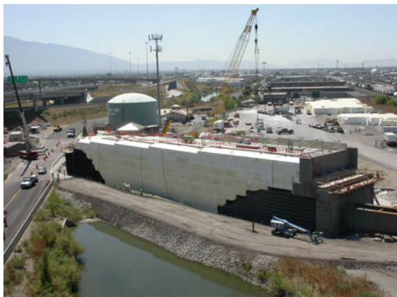
Fig. 1 Free-standing EPS embankment for light-rail train system, Salt Lake City, Utah, USA
