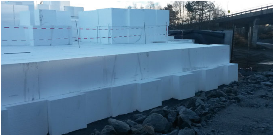
Fig. 6 EPS filling at the end part of the abutment filling—ready to be connected to the next EPS filling
