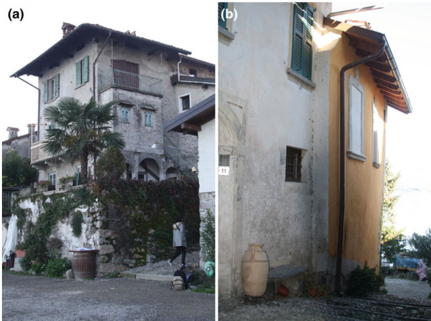
Fig. 4 Isola Superiore or Pescatori, houses needing a restoration plan: a the old primary school and b a 18th cent. private house with inflected walls
