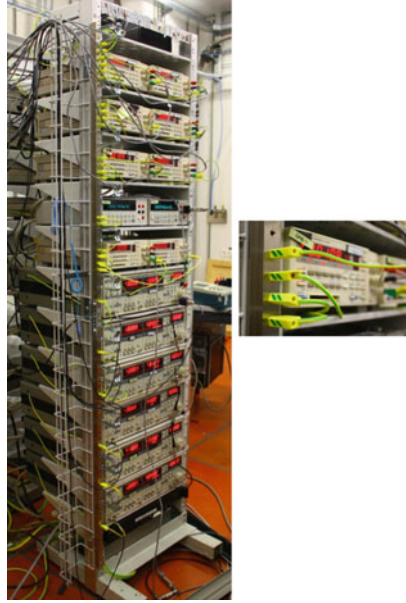
Fig. 7.9 New rack design with low-impedance ground connections for all measurement devices
