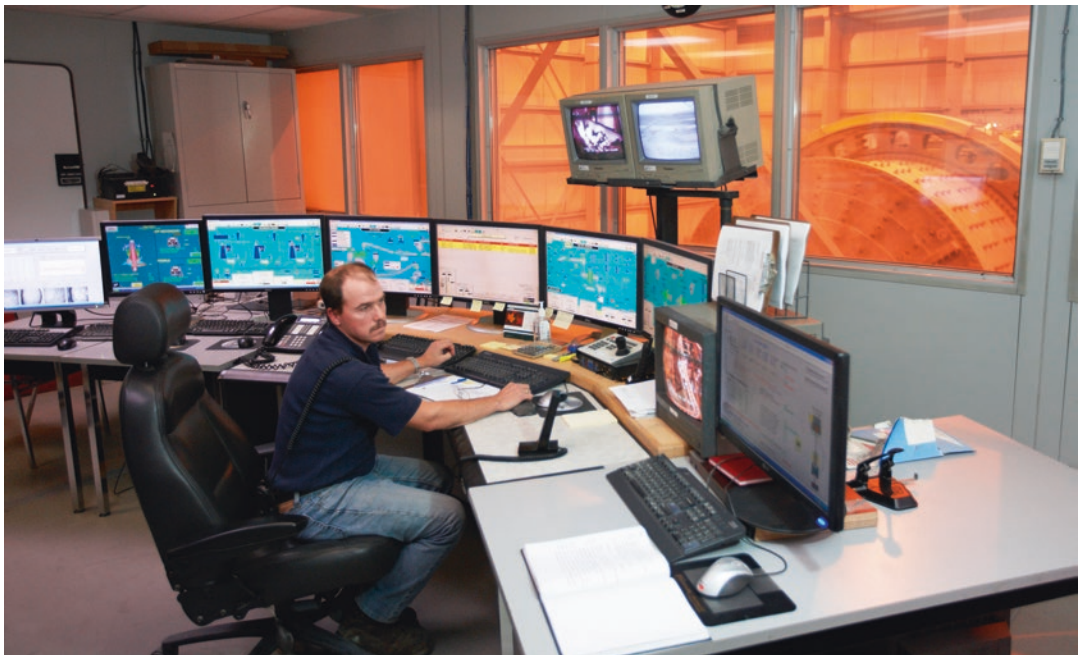
■ Fig. 6.26 Mill control room (Image courtesy of North American Palladium Ltd.)
