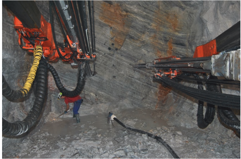
■ Fig. 5.77 Two-boom drilling rigs performing face drilling (Spain) (Image courtesy of Magnesitas de Rubián, S.A.)
