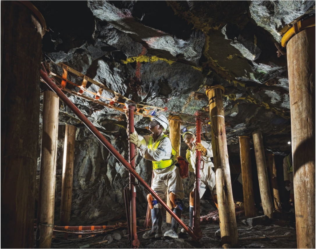
■ Fig. 5.57 Installation of canopy jack at Tumela Mine (South Africa) (Image courtesy of Anglo American plc)
