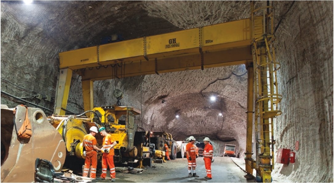
■ Fig. 5.48 Station for underground maintenance equipment (Spain) (Image courtesy of Iberpotash)
