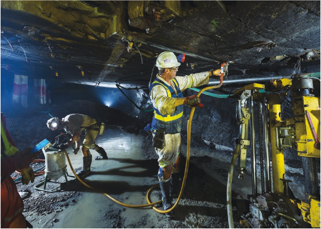
■ Fig. 5.54 Installing rockbolts at Bathopele mine (South Africa) (Image courtesy of Anglo American plc)
