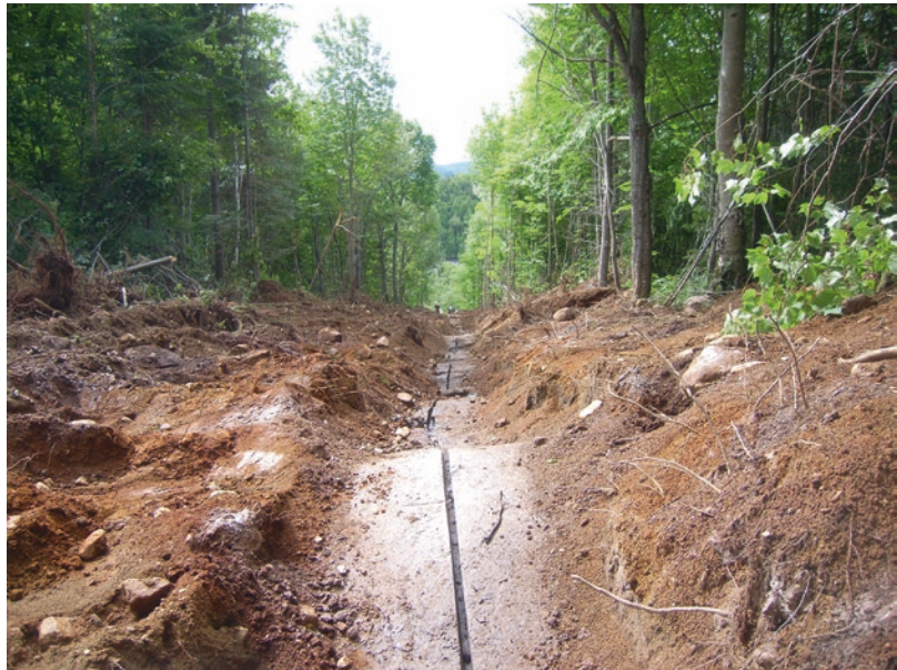
■ Fig. 3.73 Part of a trench including a channel sampling (Image courtesy of Nouveau Monde Mining Enterprises Inc.)
