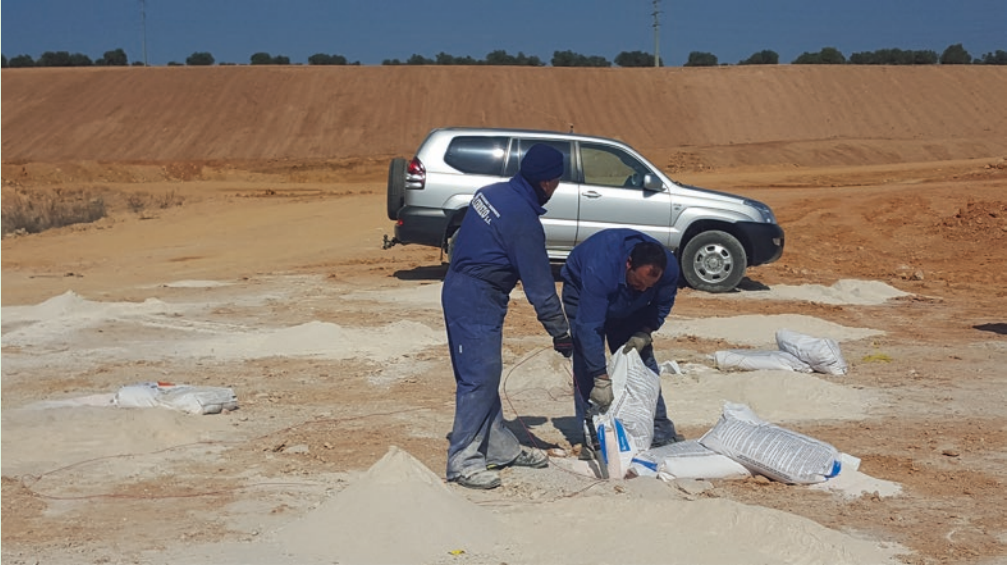
Fig. 5.80 Loading operation of ANFO nylon bags (Image courtesy of Octavio de Lera)
