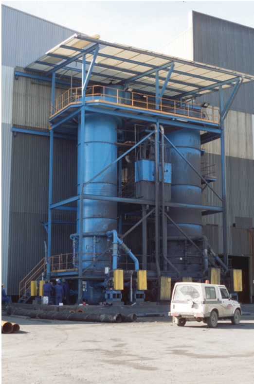
■ Fig. 6.67 Column flotation cells
