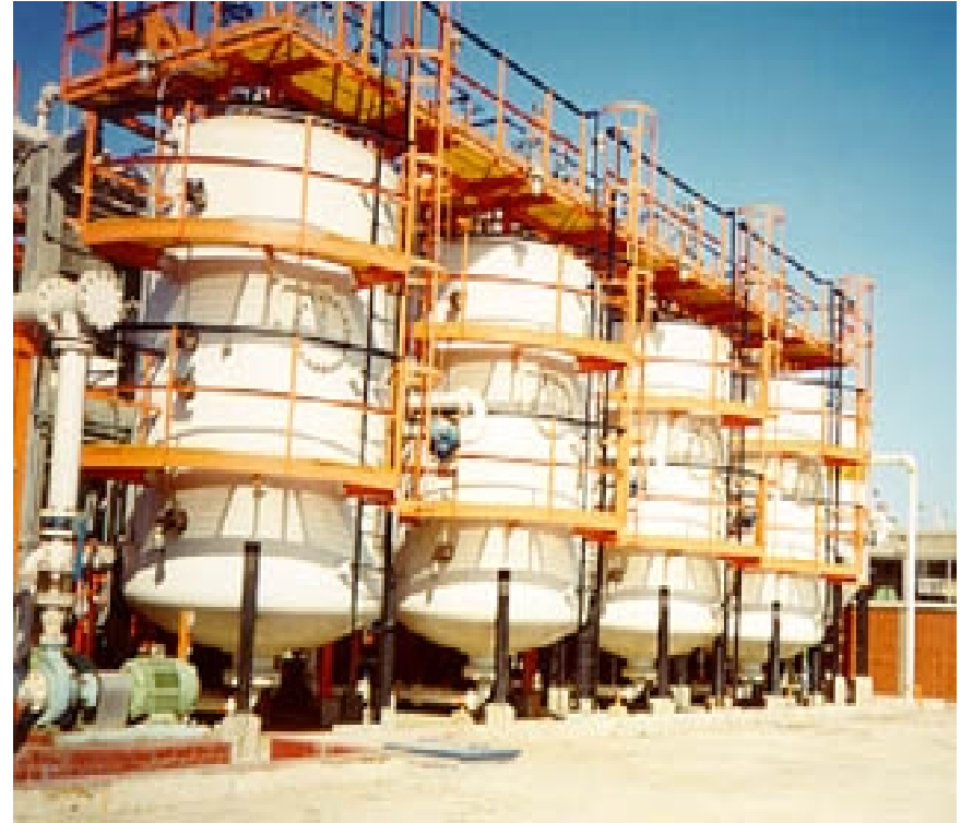
LARGE-SCALE ION EXCHANGE COLUMNS
