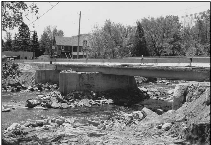
Figure 4.11 It's time for this solid wall pier, located in a stream crossing, to be replaced.
