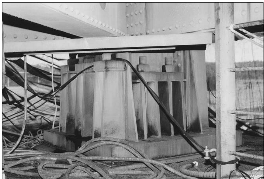
Figure 4.19 Some bearings, like the one shown above, can be quite massive in size.
