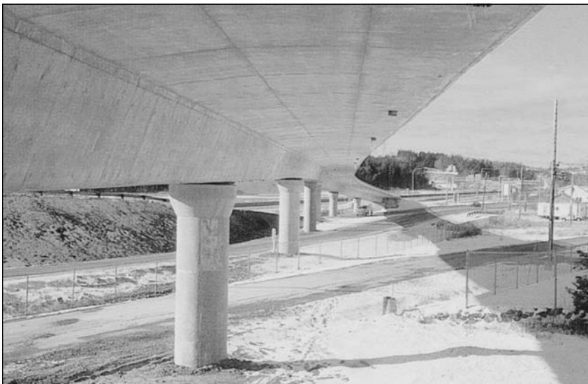
Figure 4.7 A series of single column piers support a prestressed concrete bridge. (Photograph courtesy of D. S. Brown Company, North Baltimore, Ohio.)
