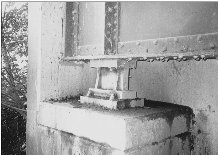
Figure 2.5 This bearing and pedestal are in good condition.
