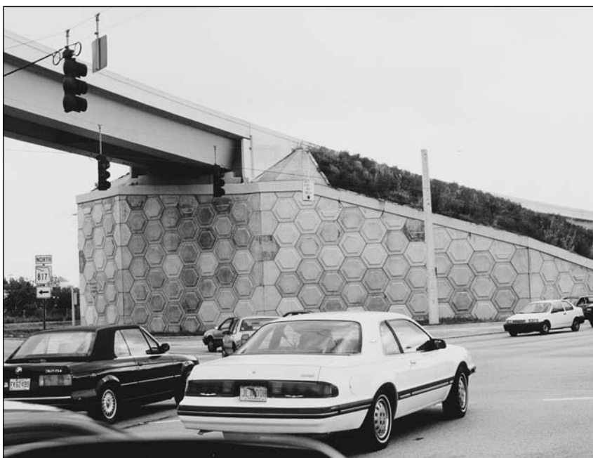
Figure 4.2 A reinforced earth abutment is used to support this composite steel bridge.
