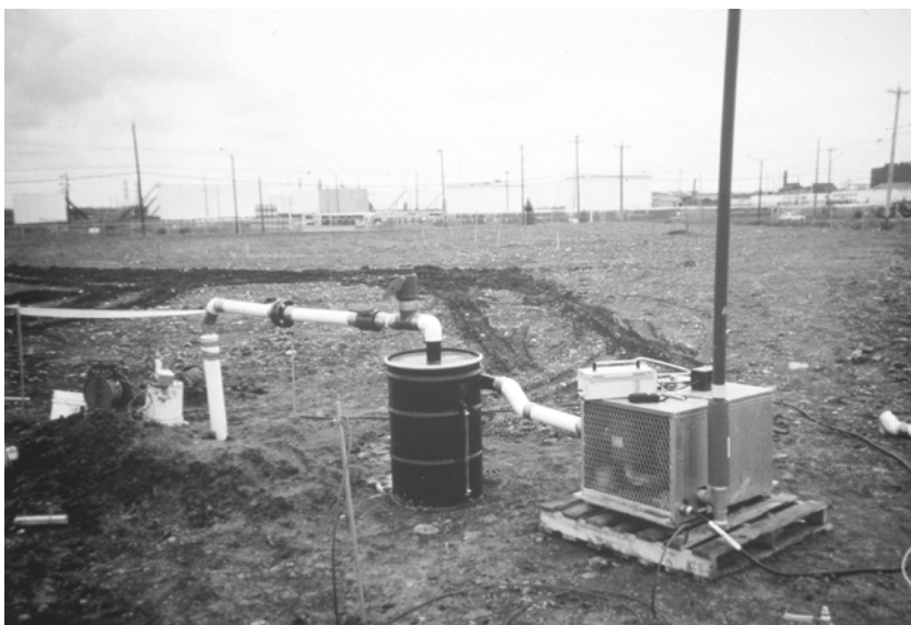
FIGURE 3.16 Prepilot-test setup for soil vapor extraction: well head, knock-out drum, suction blower. Monitoring wells are just outside the photograph to the left and right.
