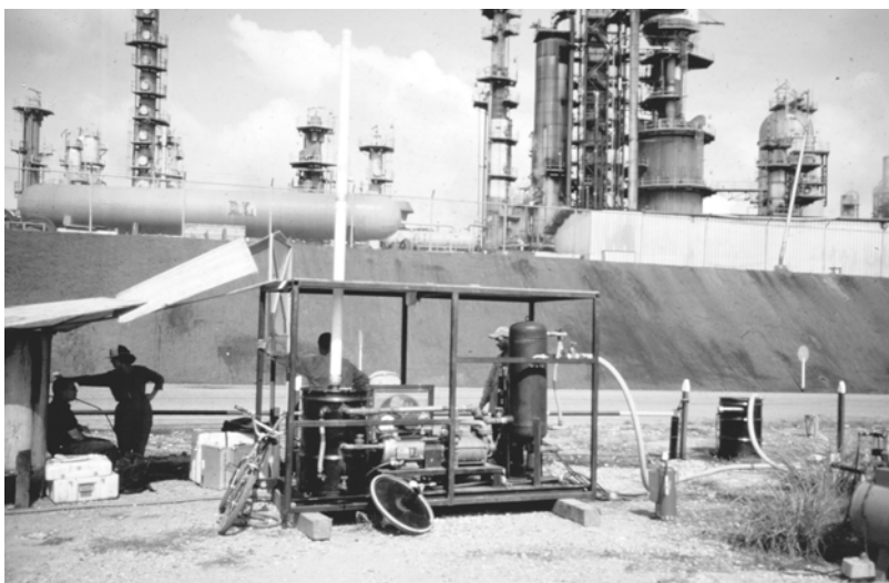
FIGURE 3.19 Pilot multiphase extraction unit at the site, with refinery complex in the background.
