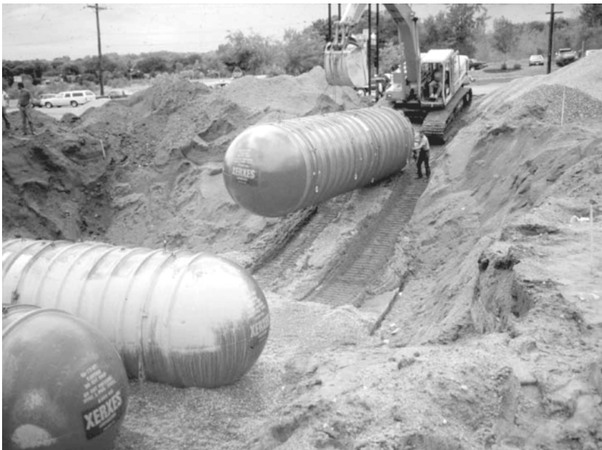
FIGURE 3.2 Petrol service stations are a common sight at street corners and along roadways the world over. Fuel stored in underground tanks may leak into surrounding soils and eventually impact groundwater. (Courtesy of Komex.)
