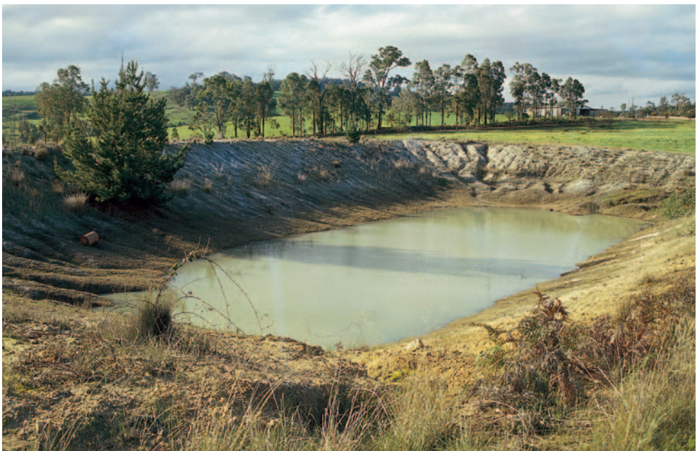
b) A failed dam in Western Australia, built with uncompacted dispersive clay that only holds water to the undisturbed level below. The pine tree growing at the highest possible water-holding level indicates how rarely the water rises to this point.
