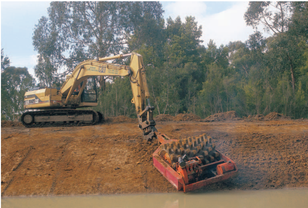
b) A sheepfoot roller with a self-contained vibrating motor, manoeuvred by an excavator over a slick clay wall where other machinery could not safely operate.
