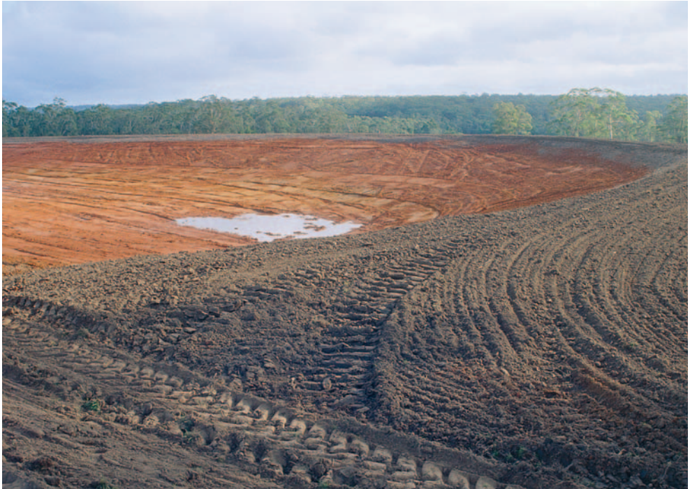
a) Newly constructed dam with topsoil replaced only on the highest levels.
