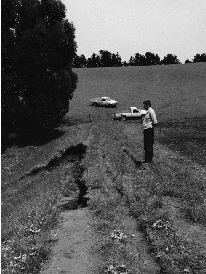
Photo 6.2 Slump extends to the centre-line of the embankment.
