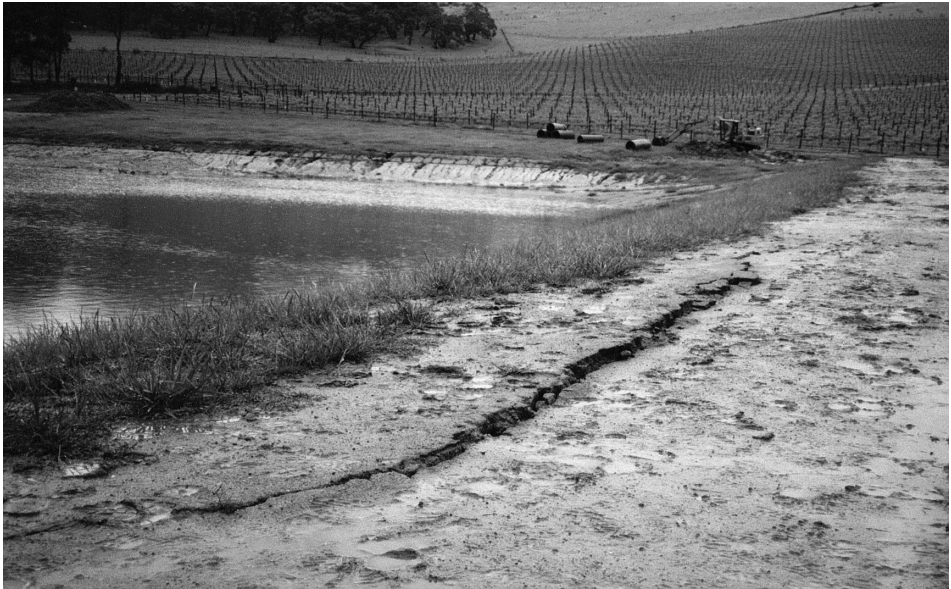
Photo 6.1 Longitudinal cracks on the crest of the embankment (Source: B. Lewis).
