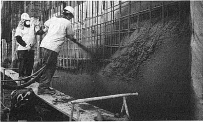
Fig. 4. Thick sections should be built up in layers sloping to the face at an angle of about 45 degrees. The surface should also be sloped longitudinally to resist rebound entrapment.
