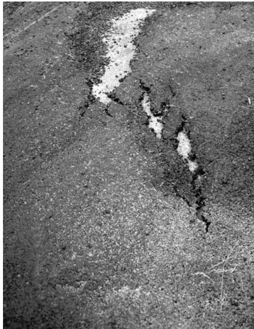
FIGURE 11.32 An example of the tearing of an SMA mat due to the lack of a tack coat on the cement concrete bottom layer. (Photo courtesy of Krzysztof Błażejowski.)
