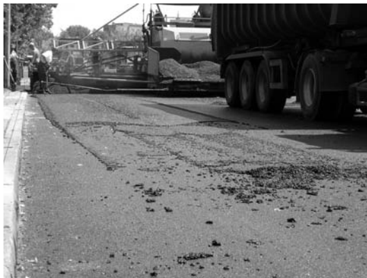
FIGURE 11.33 Remains of mixture left on a bottom layer resulting in unevenness of the finished course. (Photo courtesy of Krzysztof Błażejowski.)
