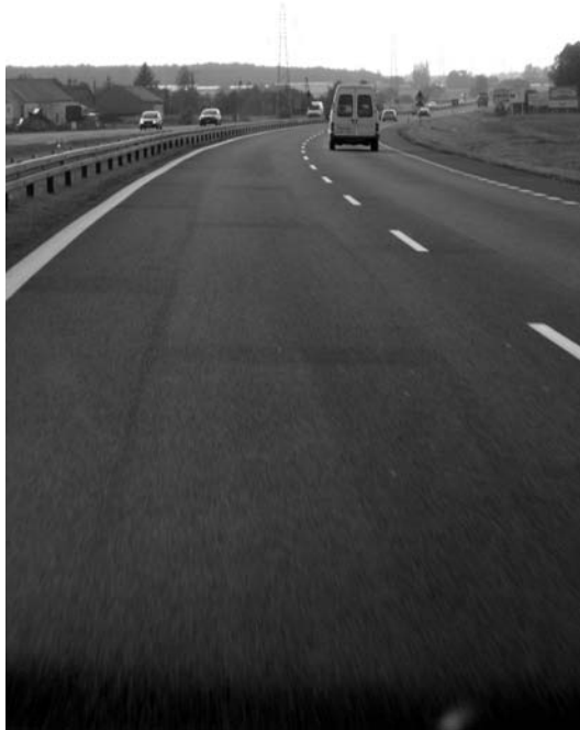
FIGURE 10.16 Movement traces of a roller after gritting a freshly made SMA layer. (Photo courtesy of Krzysztof Błażejowski.)
