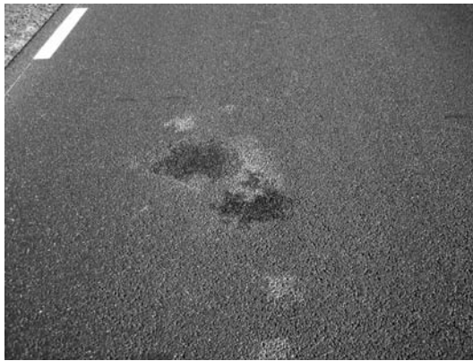
FIGURE 11.11 Seepage of water through an SMA layer. (Photo courtesy of Bohdan Dożycki.)
