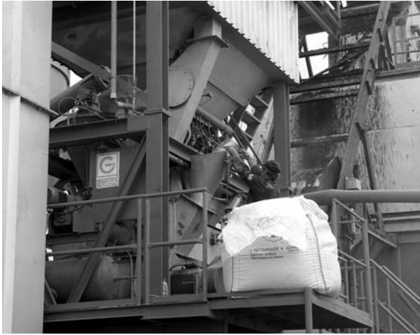
FIGURE 9.8 Manual proportioning control of a granulated stabilizer directly into the pugmill. (Photo courtesy of Bartosz Wojczakowski.)
