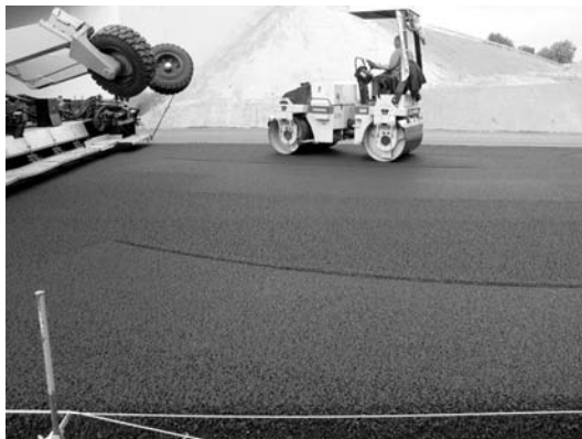
FIGURE 10.11 The particular way rollers approach the paver, with a turn being made right behind the paver. (Photo courtesy of Konrad Jabłoński.)
