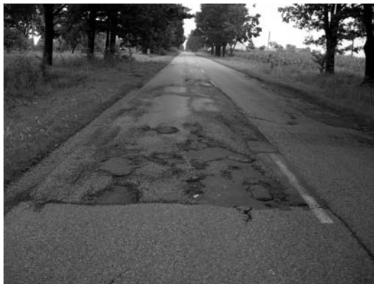
FIGURE 11.25 Beginning of a work site—effect shown years later, a consequence of spreading too cool a mixture at the beginning of the work site. (Photo courtesy of Krzysztof Błazejowski.)
