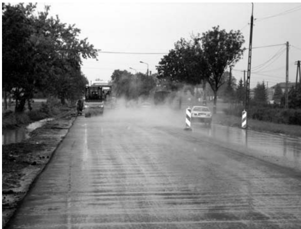
FIGURE 10.4 Laying down SMA during rainfall is not a desirable (and is mostly a forbidden) practice. (Photo courtesy of Krzysztof Błażejowski.)
