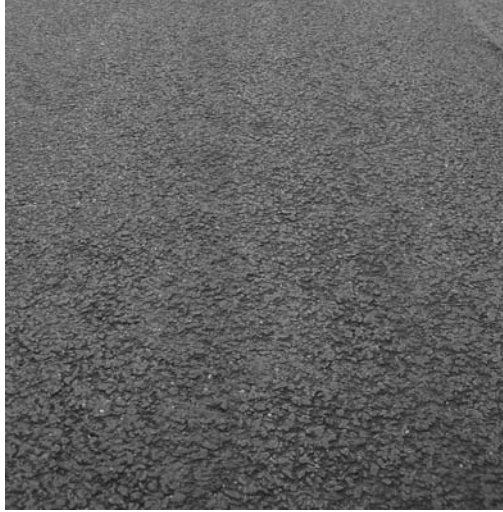
FIGURE 11.10 The surface of an SMA course just after spreading at too low a temperature. (Photo courtesy of Krzysztof Błażejowski.)
